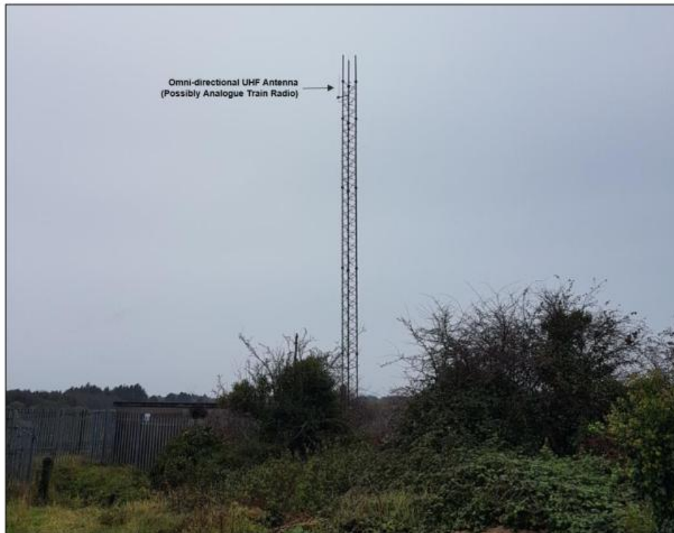
Plate 15-1 Telecoms Mast at Claremorris Train Station
